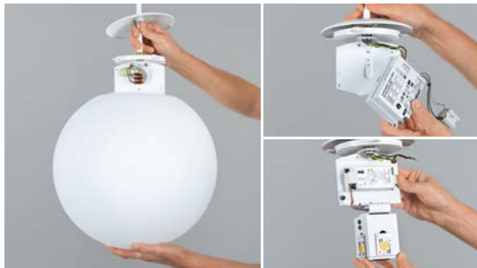
Conversion of a pendant luminaire with compact fluorescent lamp to LED
